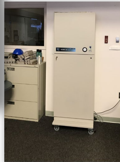
Installed Portable & Permanent Air Filters
