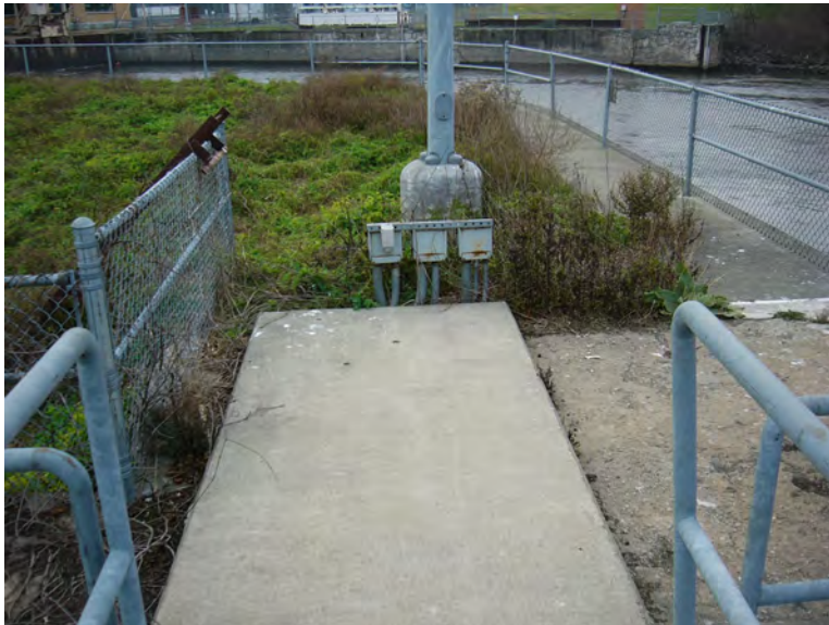
Figure 8: Power at Headrace
