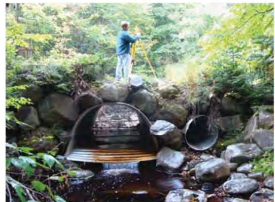
Before - a barrier to fish movement
